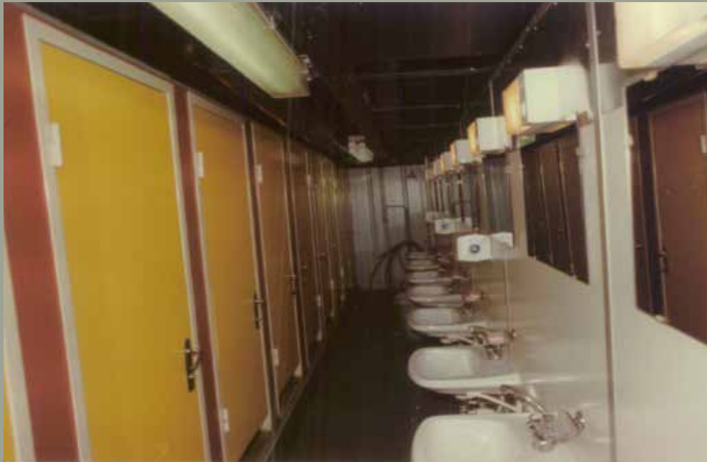
Toilets in the container section on ALK.
