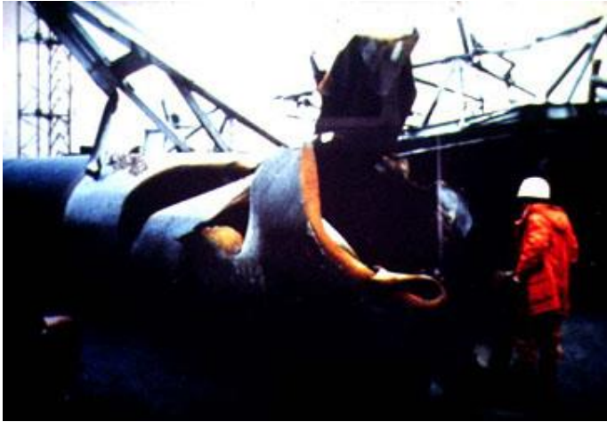
D4 brace, upper breach.
